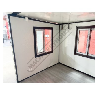
Inside 2 Has Slight Damaged Wall
