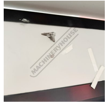
Inside 2 Has Slight Damaged Wall Close Up
