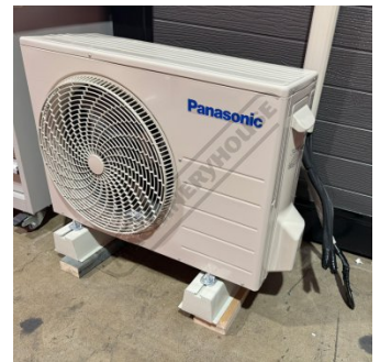
Outside AC UNIT
