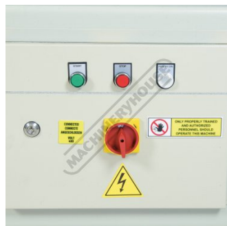
Main Power Control Panel & Isolation Switch
