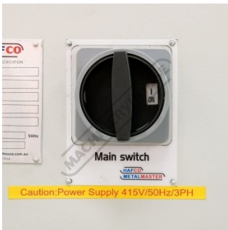
Main Isolation Switch
