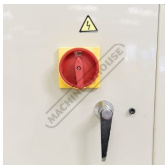
Main Isolation Switch
