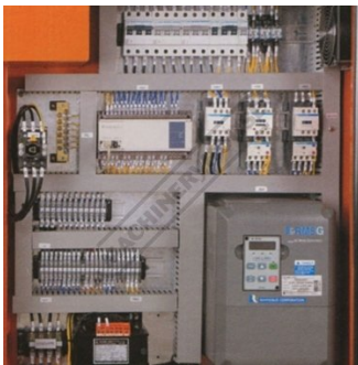
Electrical Control Cabinet
