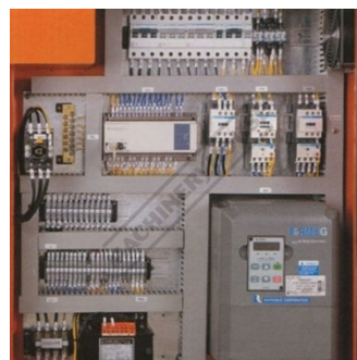
Electrical Control Cabinet
