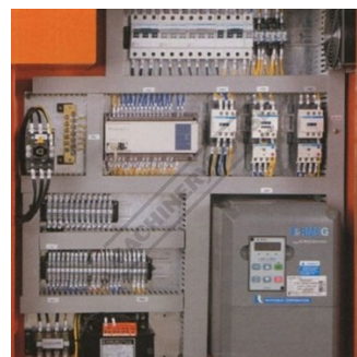
Electrical Control Cabinet
