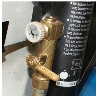
Down Feed Control
