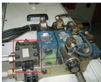
4HS9507 PILOT CHECK VALVE.2
